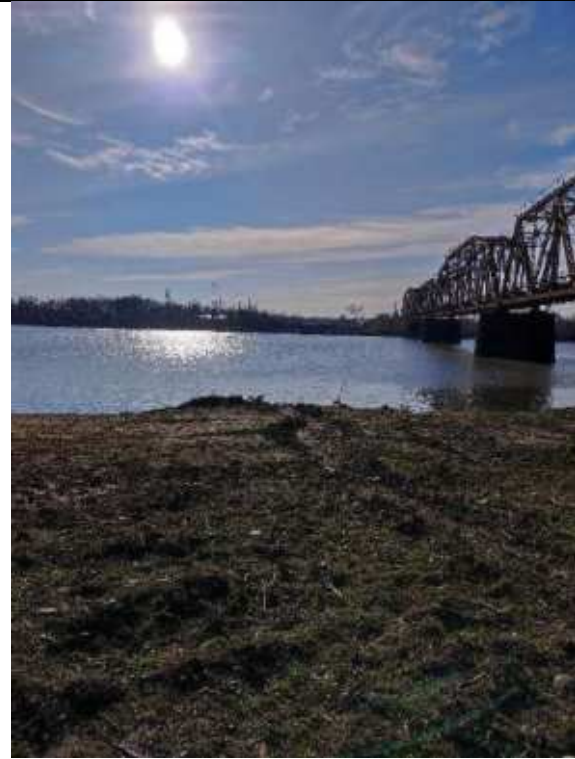
The Project view from the bridge pier location near the Rioni river
