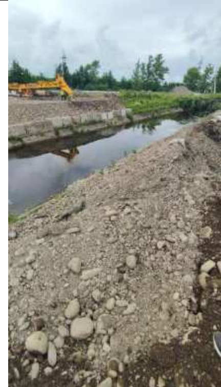
Poor soil embankment management near the amelioration canal
