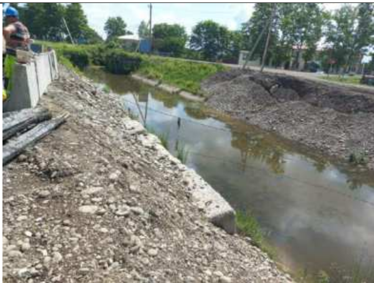
Poor soil embankment management near the amelioration canal
